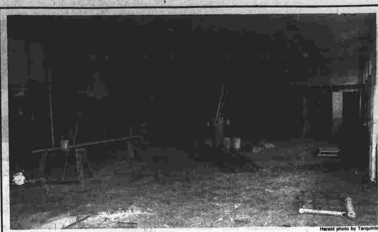
Work is progressing on the new Board of Directors hearing room in Lincoln Center, where the Sheltered Workshop used to be, but General Manager Robert B. Weiss said rising costs mean the Lincoln Center project will cost $100,000 to $200,000 more than anticipated.
